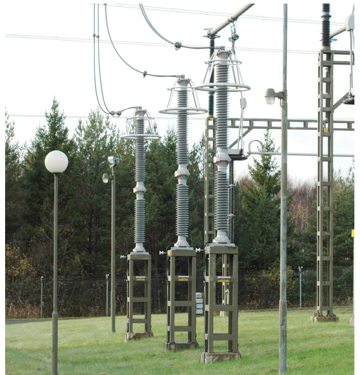
TEXLIM surge arresters connected to the line entrance
